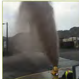
Black water from a fire hydrant
