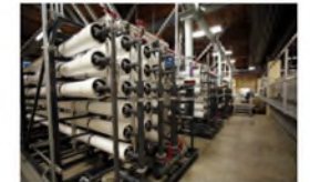
Photo: Reverse Osmosis Unit
