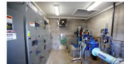
Photo: Well Pump House
